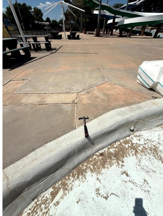
Voids around Pool
