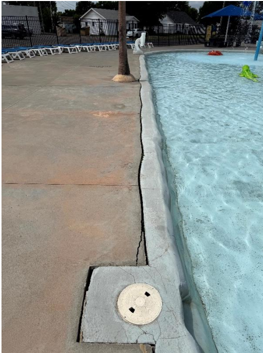
Cracking Along Deck
