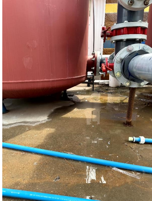
Water in Filter Area
