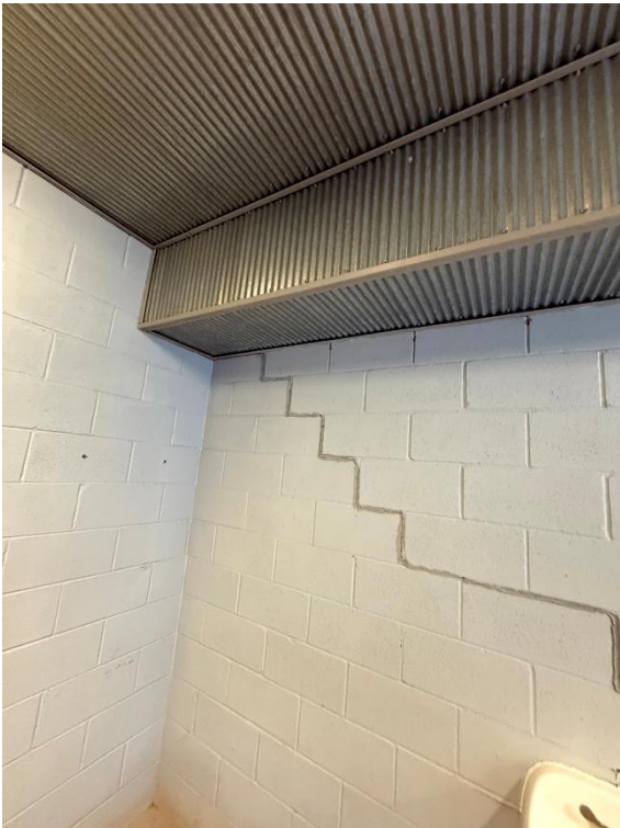
Cracking in CMU
