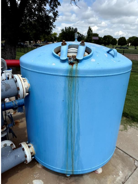
Rust on Filter
