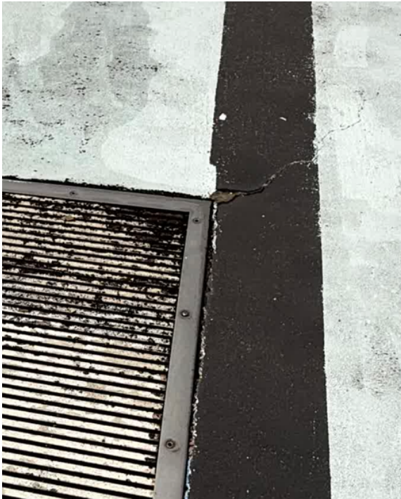
Lap Pool – Crack at Inlet
