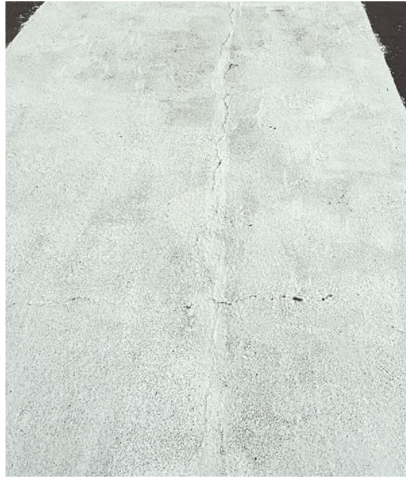
Lap Pool - Cracking
