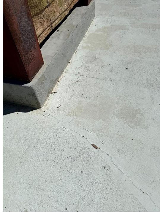
Family Pool- Crack Near Feature
