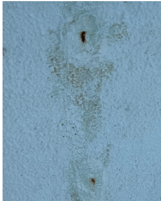
Lap Pool – Exposed Rebar
