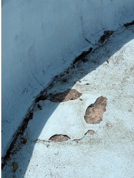
Family Pool - Spalling Concrete
