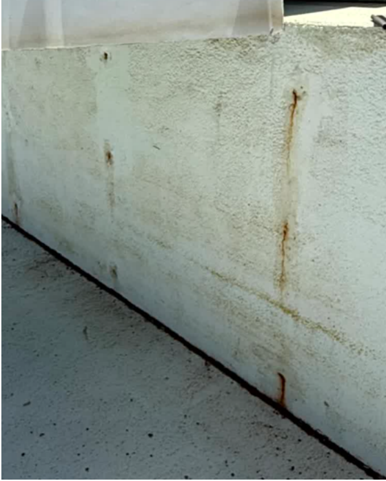
Lap Pool – Rust Spots
