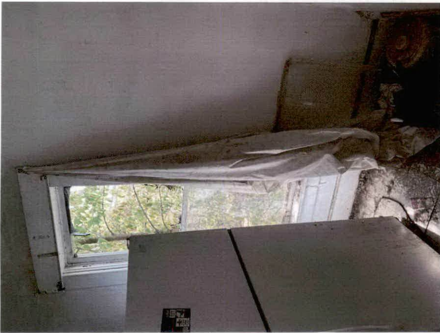
Tax Parcel #: 1493204018006000 Address: 515 N PERSHING AVE Violation #: 24-0509 Date: September 17, 2024 02:30PM
